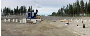
Storen Power Reserve (2024 (1) )
