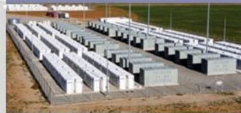
Hornsedale Power Reserve (2017)
