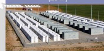
Hornsedale Power Reserve (2017)
